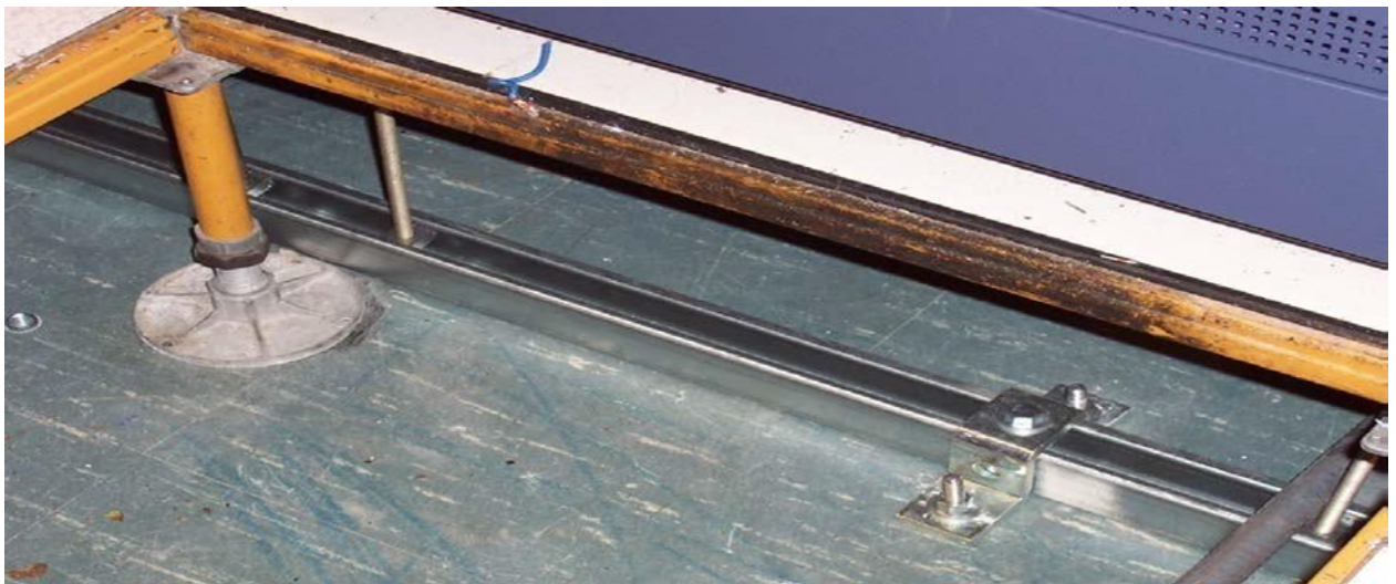
Figure 13: Cabinet and Rack Installation
